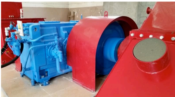
Photograph 4: Power unit - generator
