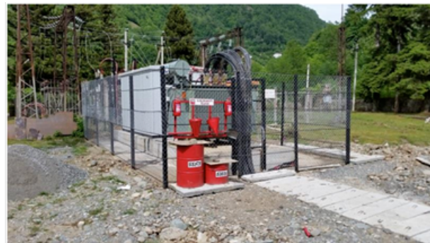
Photograph 14: New step-up transformer and fire protection
